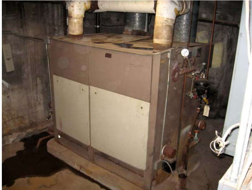
City Hall Boiler
