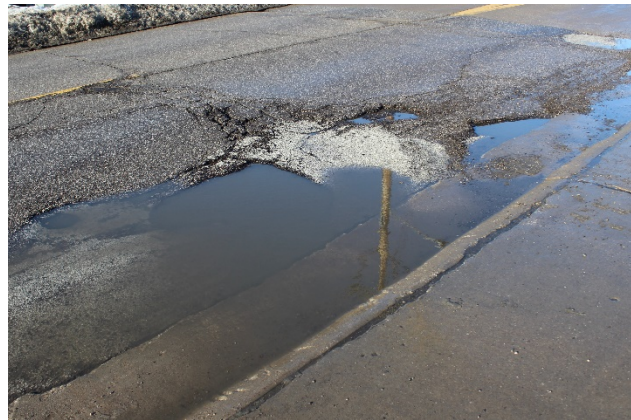
Melting snow hides the depth and width of many potholes on city streets. Drivers are urged to slow down and use caution while moving through water on the streets.
